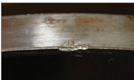
A knife crack
